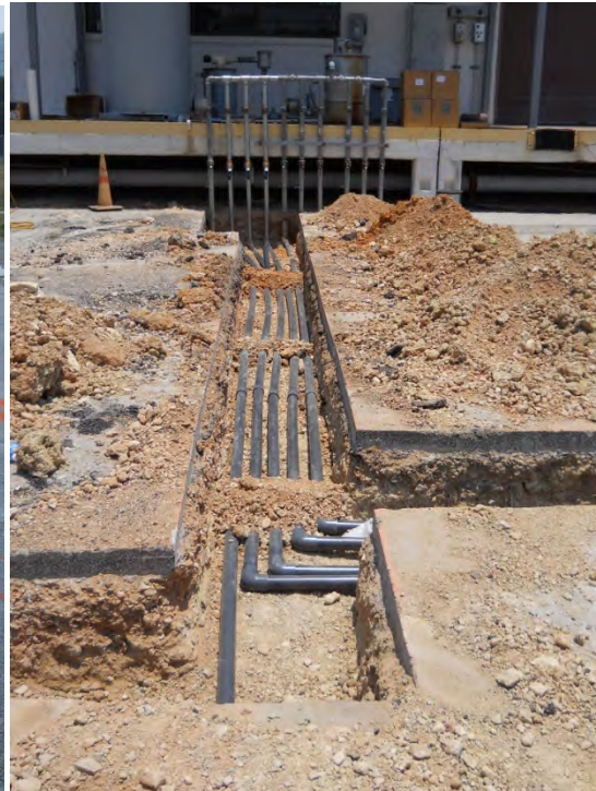
Photo 3.5- PVC lines to VEWs originating from Building 90 exterior manifold.
