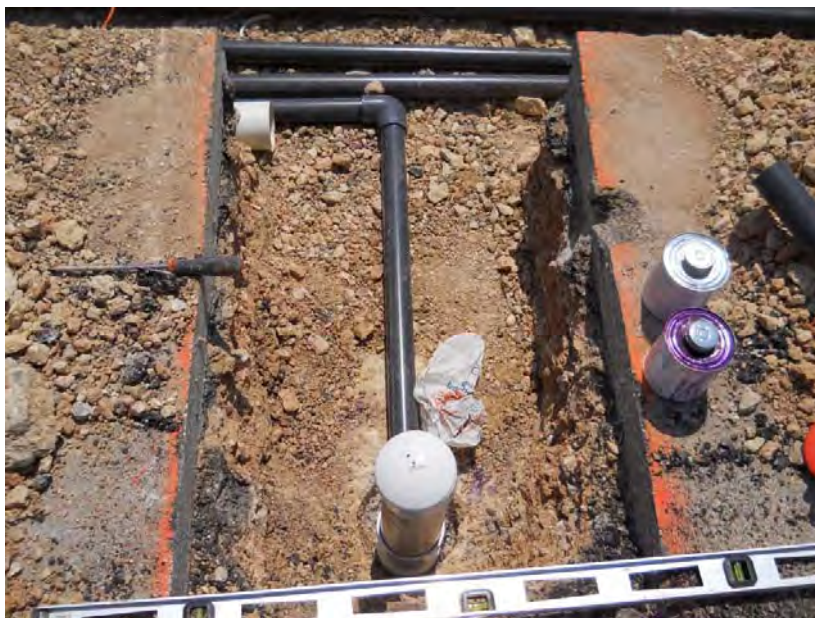
Photo 3.3 – Installation of AOC-VEW29 (photo is representative of all VEWs in this report).
