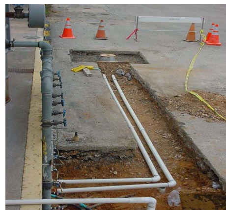
VEW 28 Piping Runs
