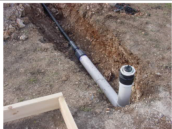
VEW Surface Piping
