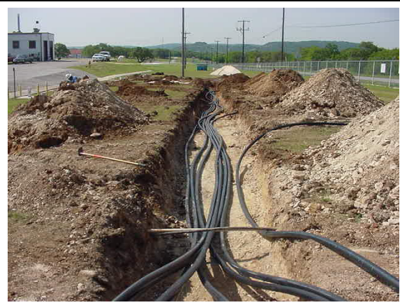
SVE Piping Runs
