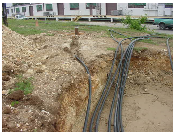
VEW 20 Piping Run
