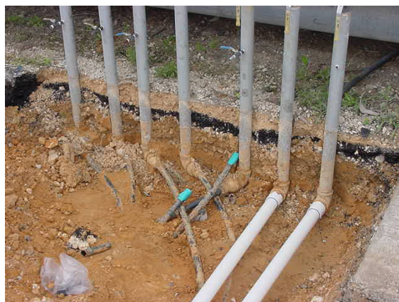
Bldg. 90 Loading Dock Connections
