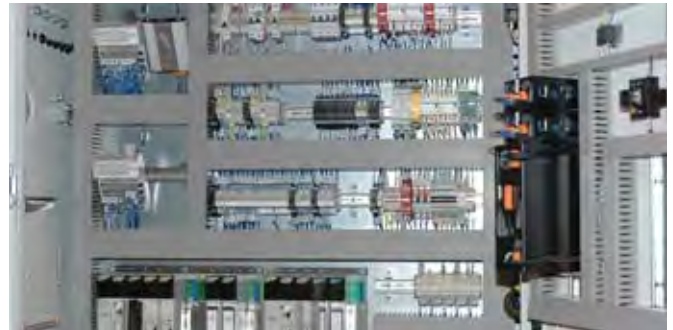
*Sample assembly showing radios, power supply, surge arrester (bottom of cabinet), terminals & relays.
