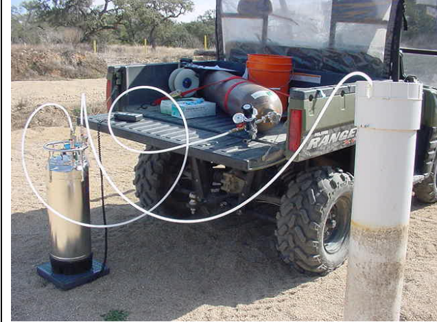
Bioaugmentation at Trench 1 sumps on 1/29/08. KB-1 canister at left, nitrogen tank in ATV, sump at right.
