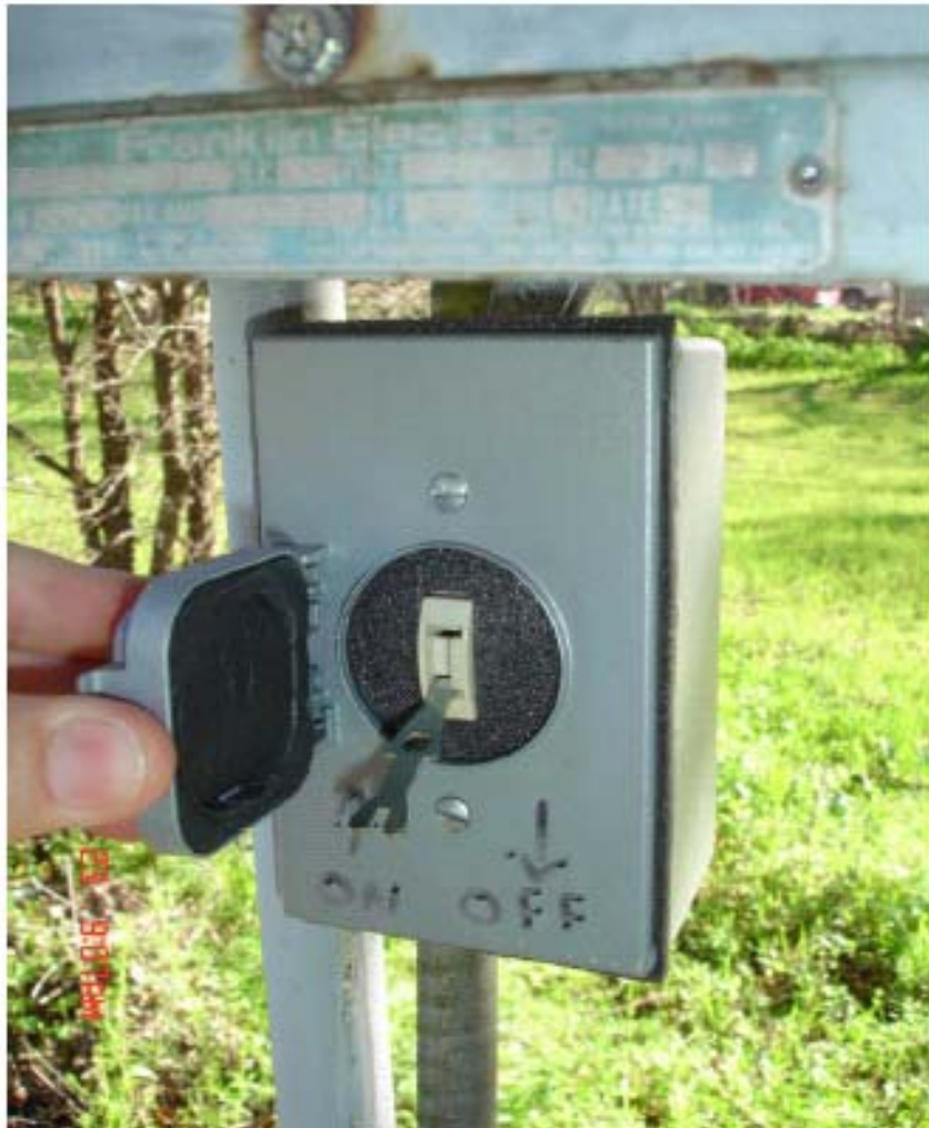
Figure Pump Switch-1
