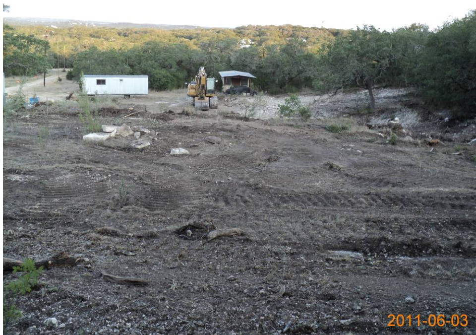
Photo 4. Preparation for excavation on top of berm at RMU-2, looking west (June 2011).
