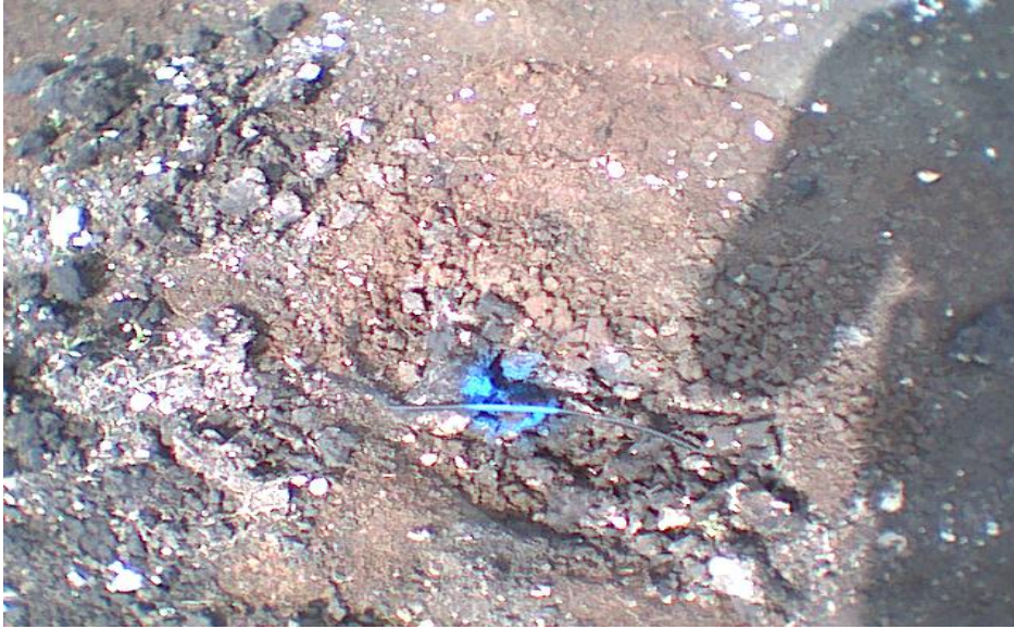
Anomaly ID LR-034 (Buried wire and concrete)
