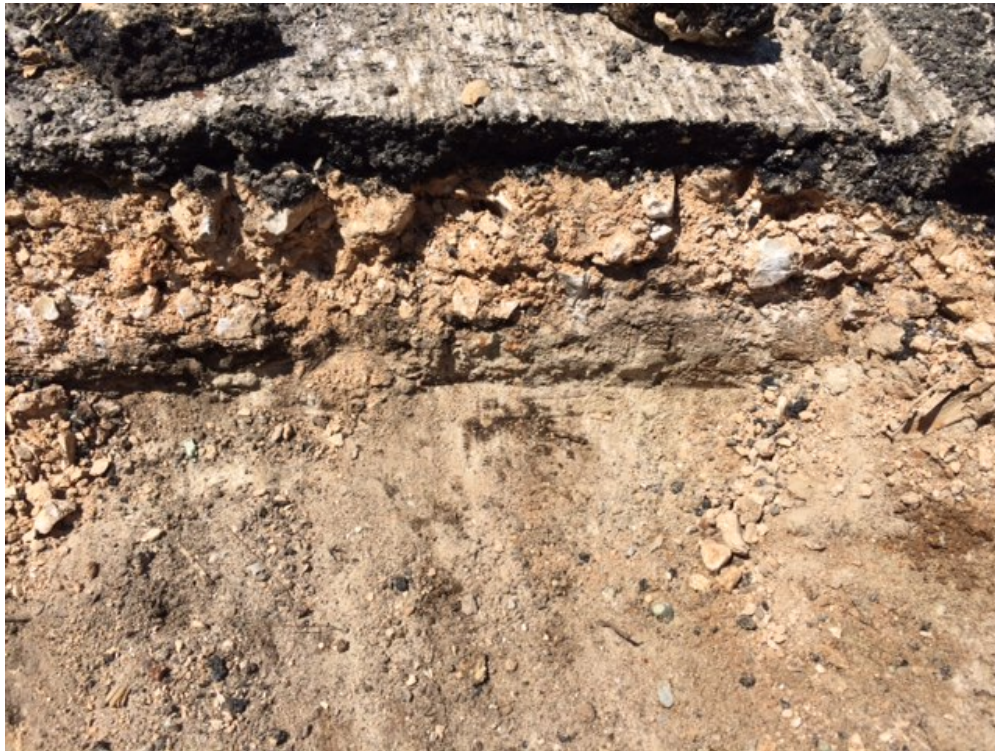
Photo 2. Sand material noted under parking lot asphalt.
