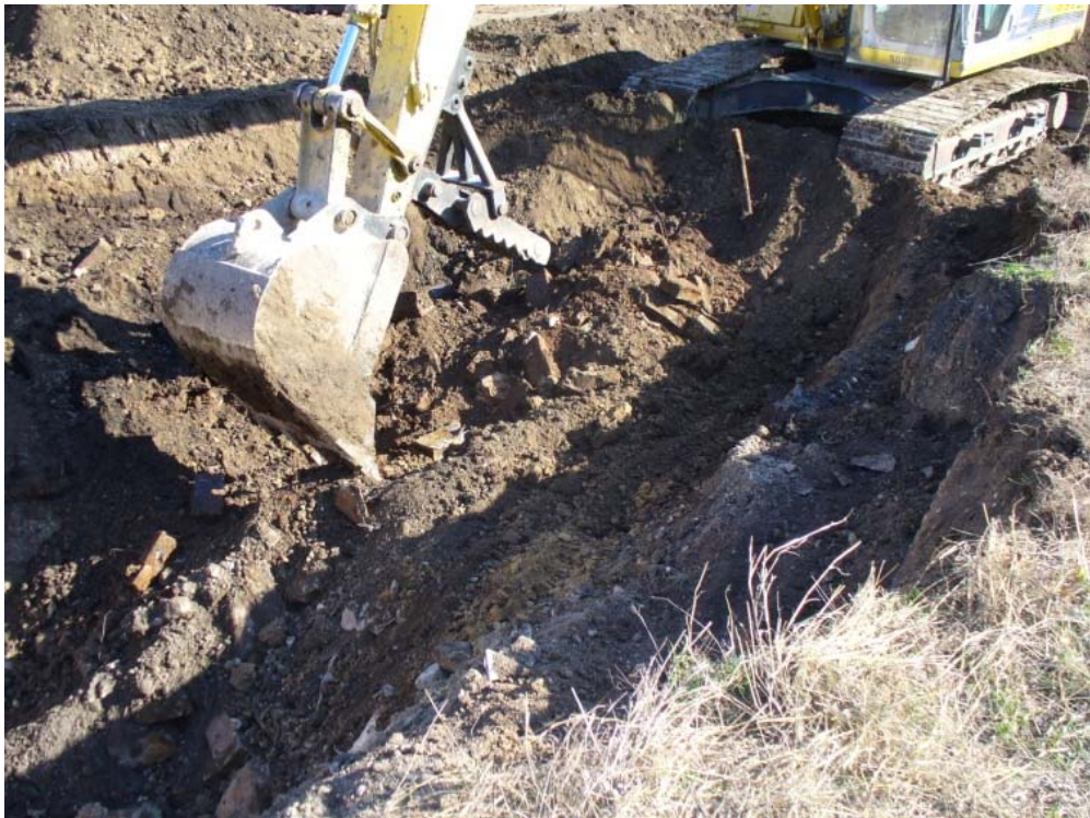
8. Top of debris in Trench A. View from west side of trench towards east, January 2011.
