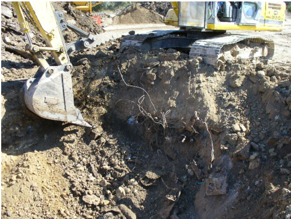
10. Excavating top of debris (steel banding, vehicle parts, misc. metal), Trench B, January 2011.
