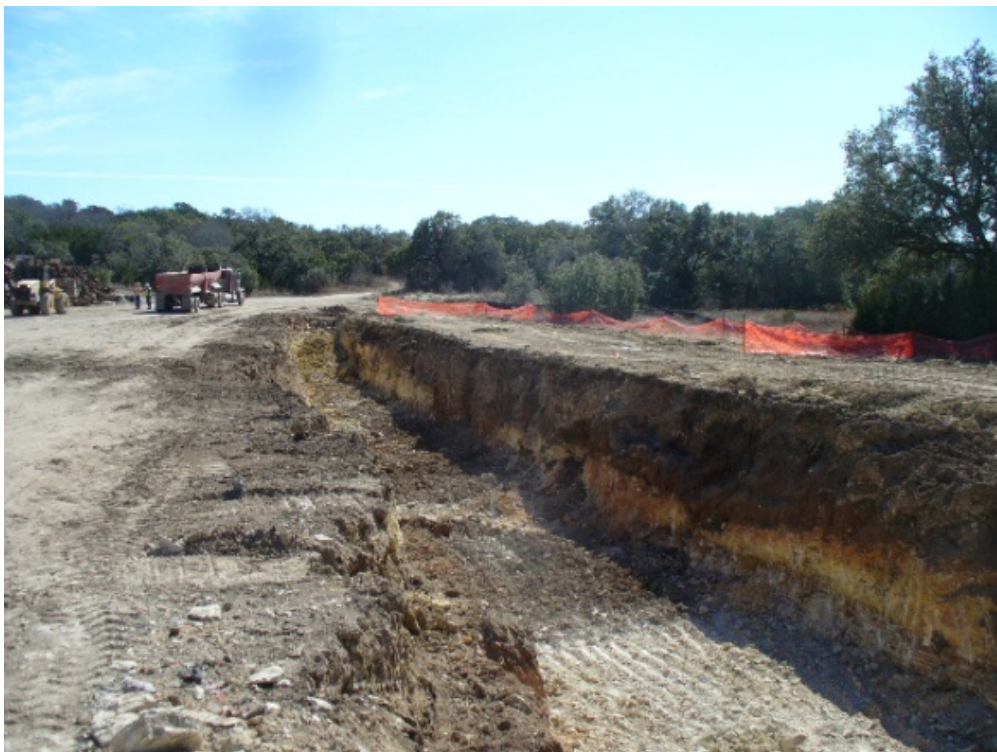
13. View of Trench B towards south. Overexcavated location B2 in foreground, January 2011.
