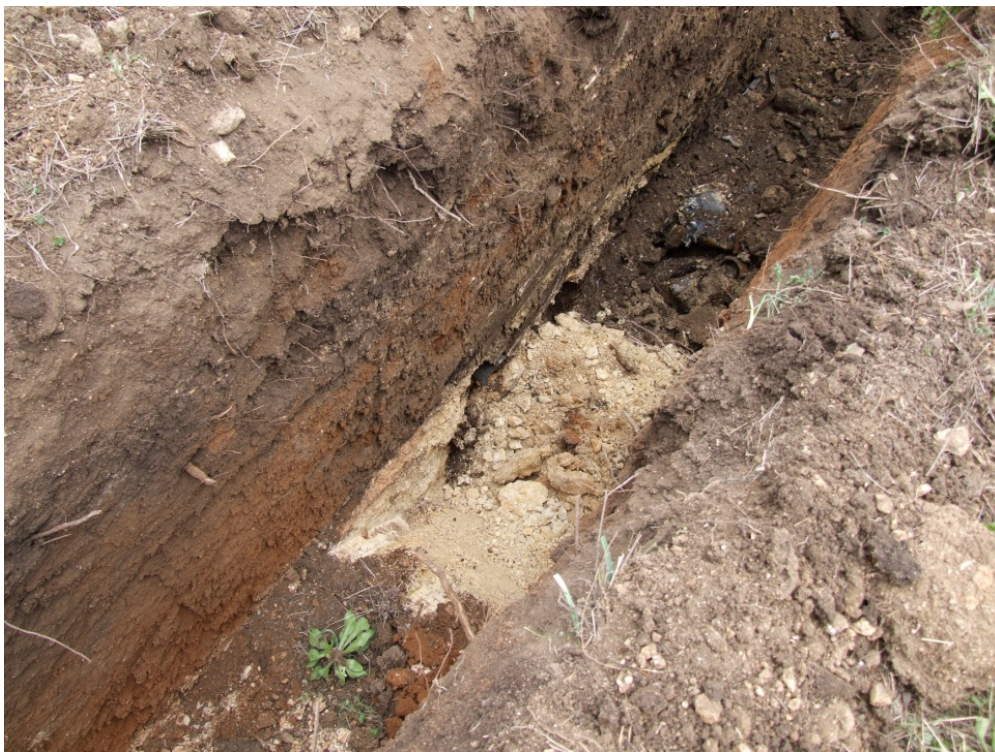
4. Close up view of top of debris in exploratory trench, April 2010 pre-IRA assessment.
