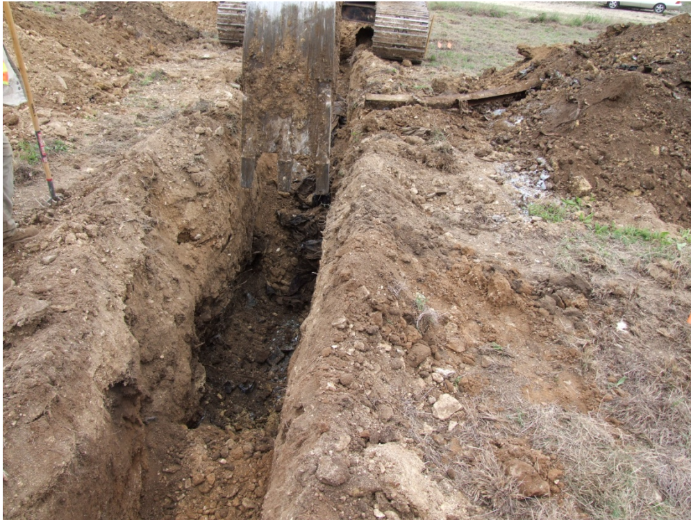
3. Interface of cover and trench debris in exploratory trench. April 2010 pre-IRA assessment.
