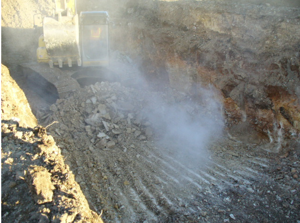
12. Overexcavating floor of Trench B at location B5. View from west sidewall, January 2011.
