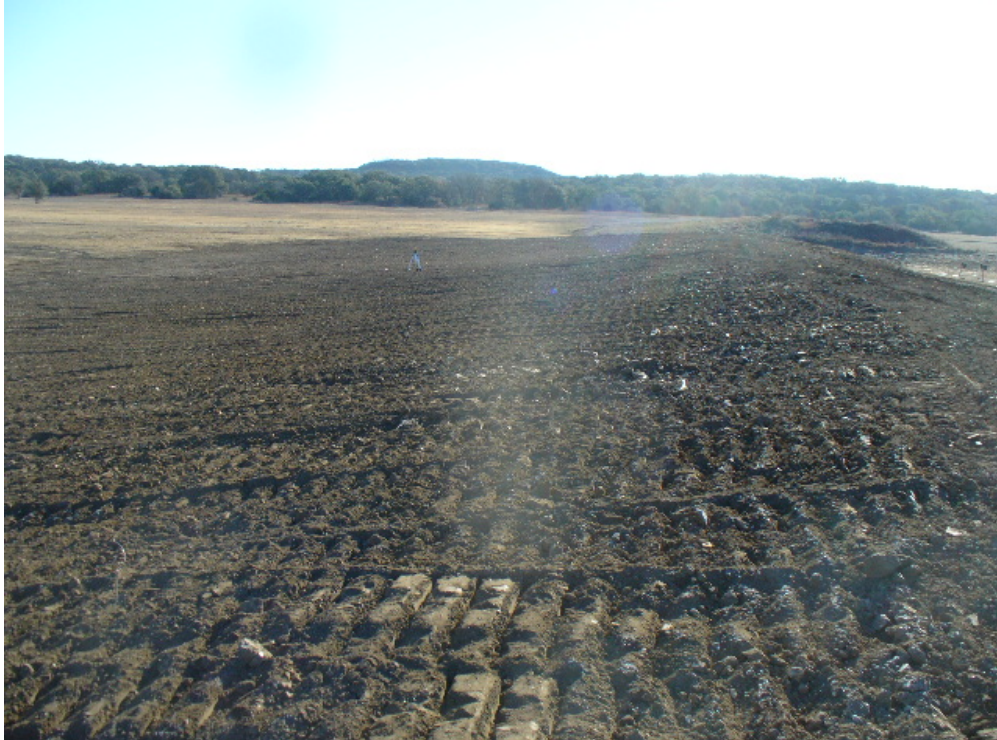
22. Final grade material placed at East Pasture firing berm March 2011. View to the east.
