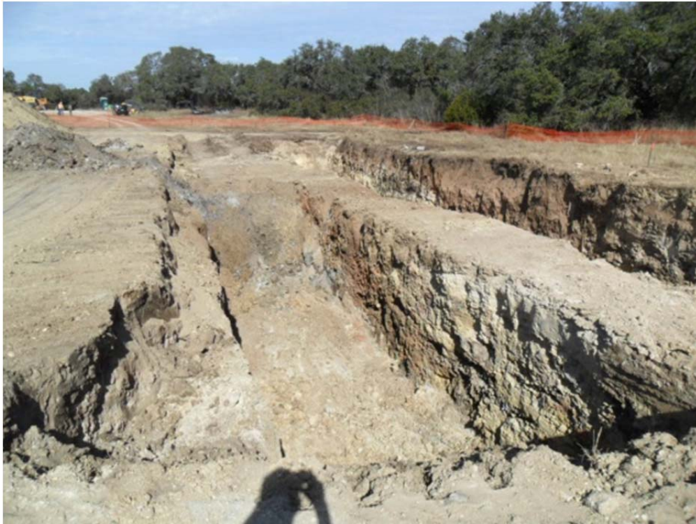
7. Southern end of Trench Cb during backfilling excavation. Note wall separating Trench Ca on right. View to north, January 2011.
