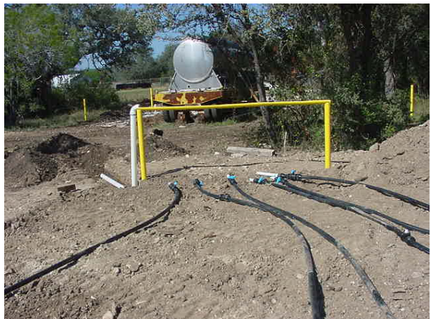
Irrigation system distribution header
