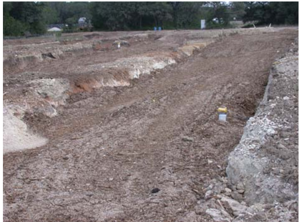
Bioreactor Monitoring Sump (Trench 5)
