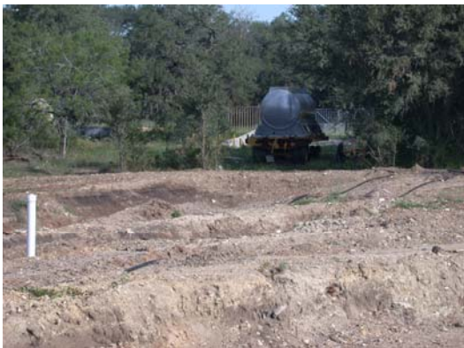
SWMU B-3 Irrigation Tank
