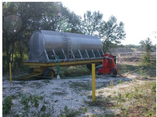
Water tank with rented pump
