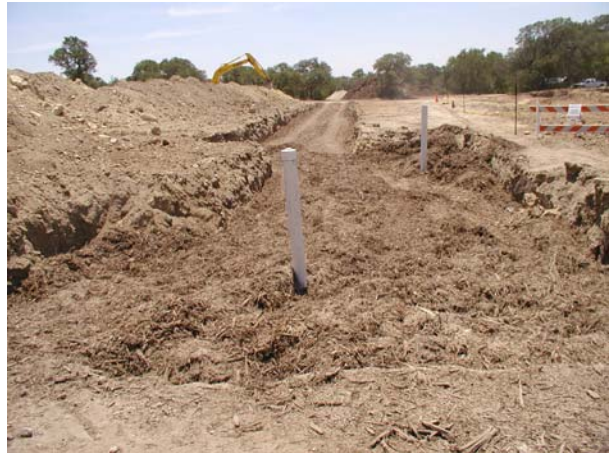
Bioreactor Monitoring Sumps (Trench 6)
