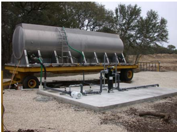
Bioreactor transfer tanks and pump
