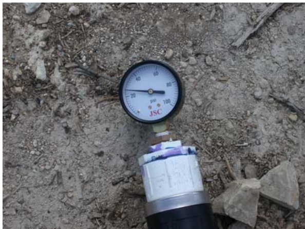
Test pressure gauge (pressure reading after nozzles)
