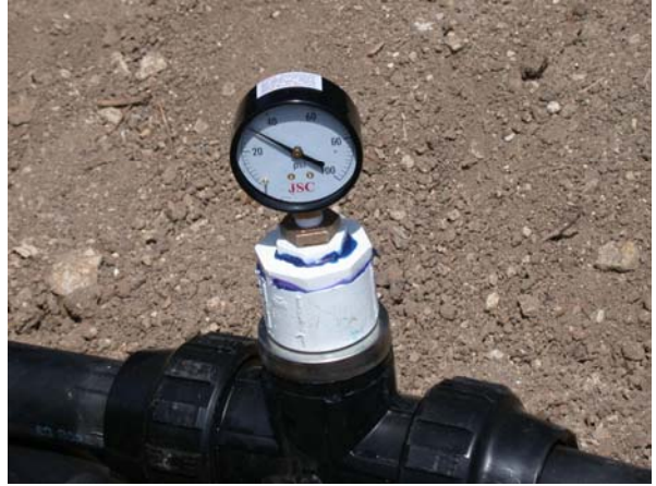
Test pressure gauge (pressure reading prior to nozzles)
