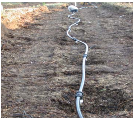
Trench 3 irrigation piping
