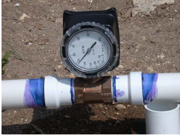
Test flow meter
