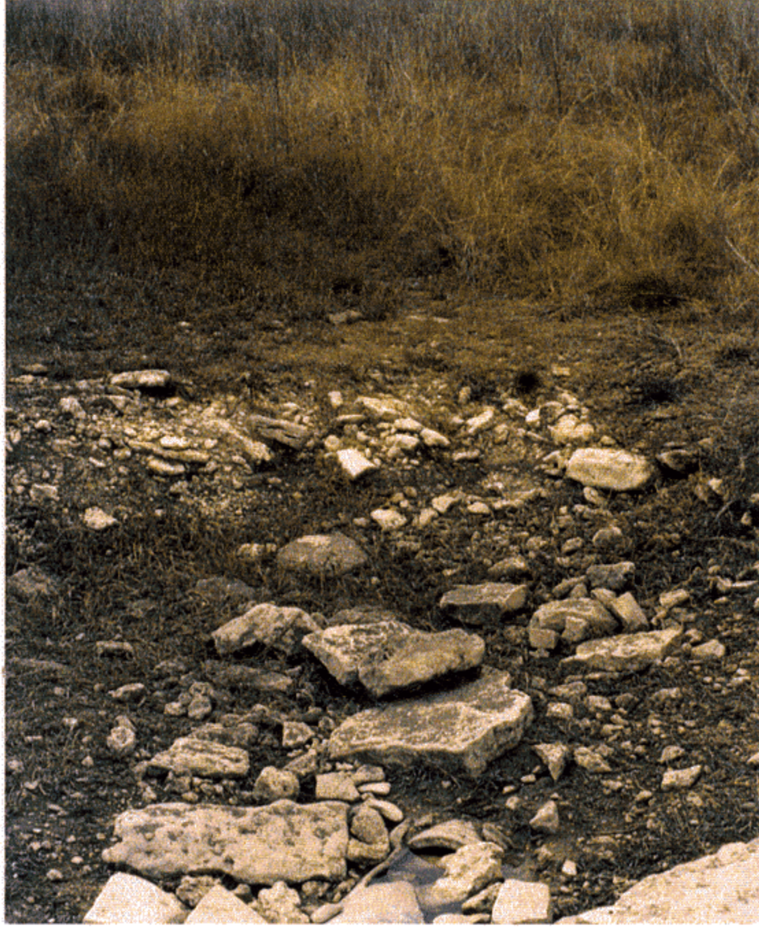
Photo 33: Broken, abandoned pipe carrying sewage approximately 300 yards downstream of motor pool leach field.
