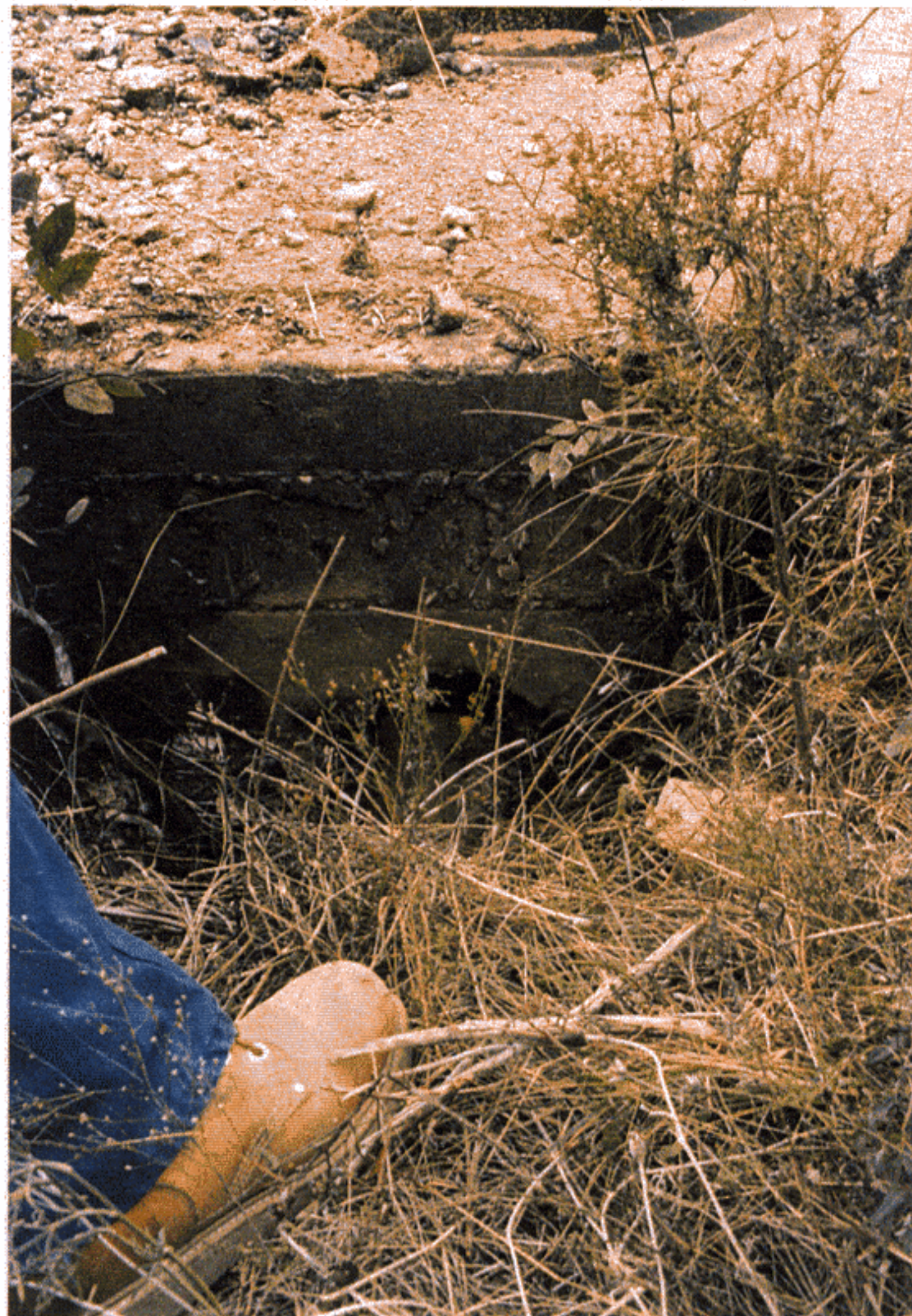
Photo 32: Broken outlet pipe from solids tank to leach field near building 45.
