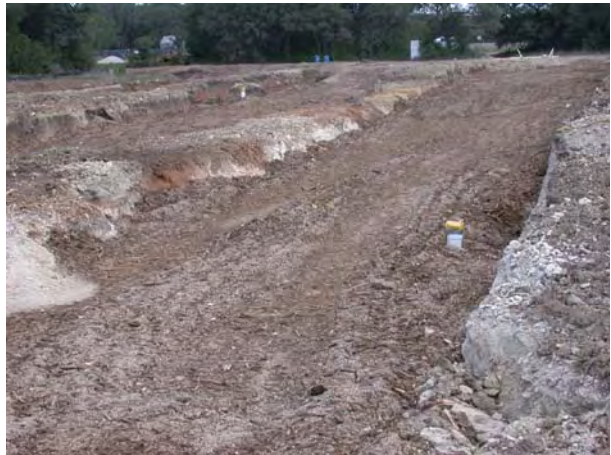
Bioreactor Monitoring Sump (Trench 5)
