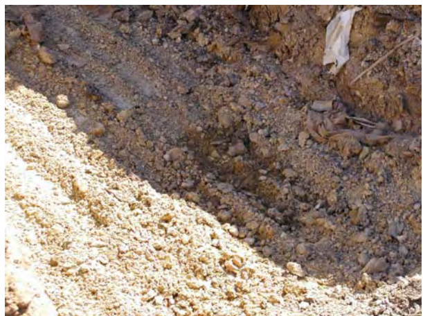
Trench 1 water infiltration
