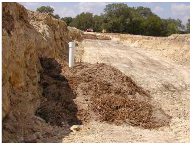
Bioreactor Monitoring Sump (Trench 5)
