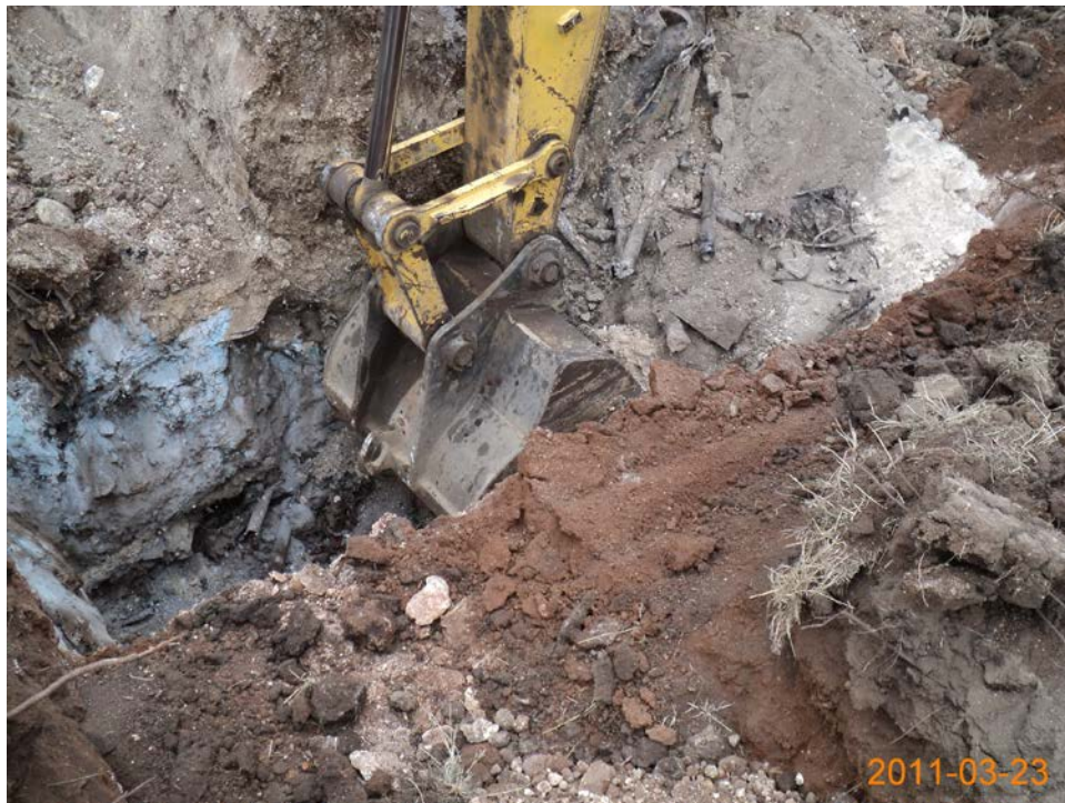
Photo 3. Light blue material found in Trench 2 at AOC-42 (April 2011).
